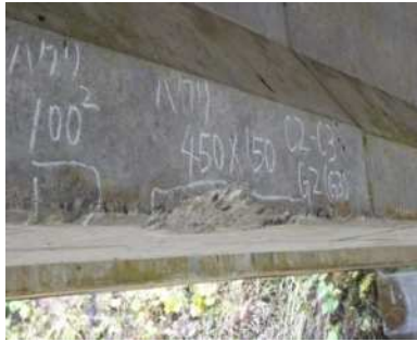
写真-主桁の欠損
